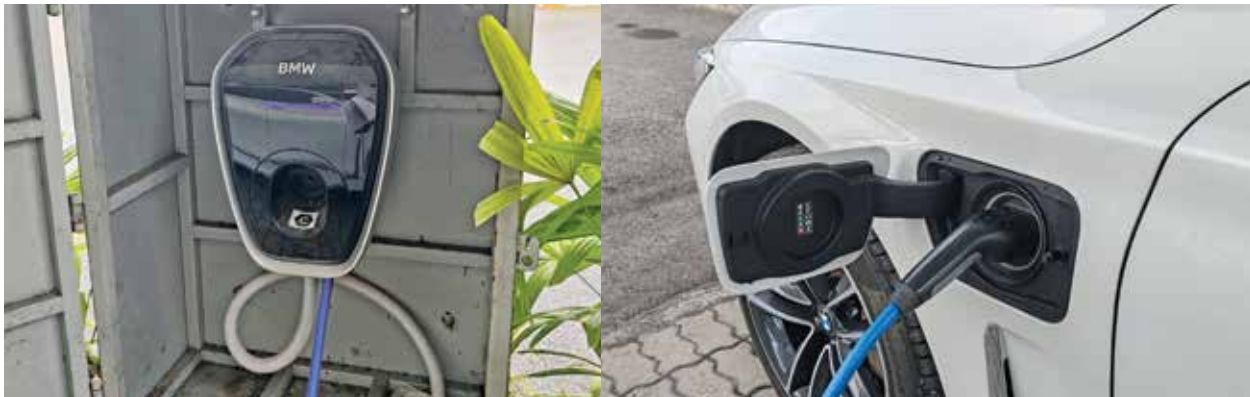
Electric Vehicle Charging Unit at our corporate office
